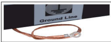
Grounding Line is provided at back side
