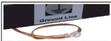
Grounding Line is provided at back side
